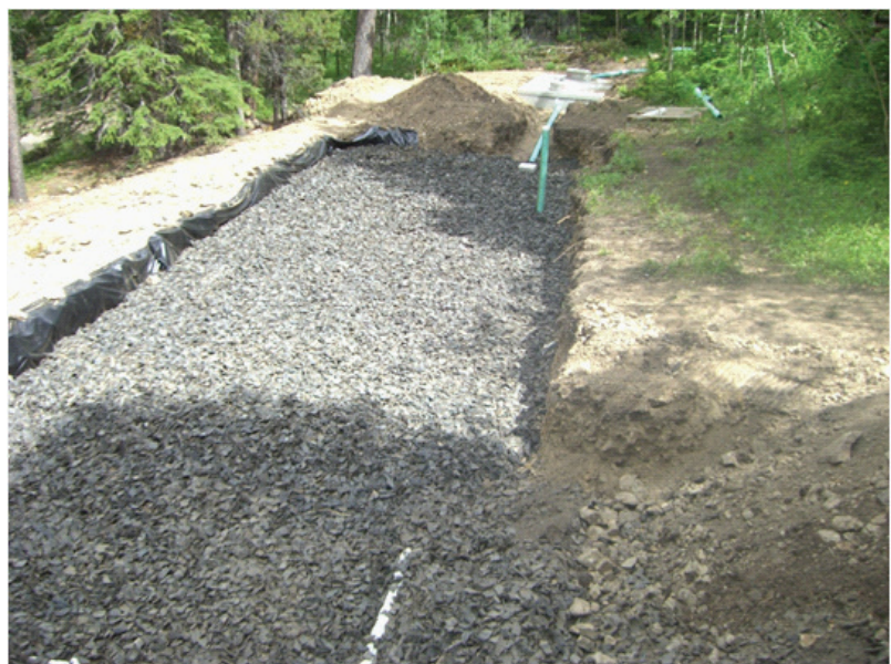
Boulder County 'Rubber Rock' Onsite Wastewater Drain Field. Tim Petz 2008.
